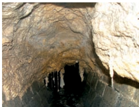
Fat beginning to block a sewer
